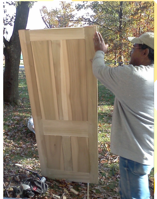
Contractor Doug Tutt prepares one of three reproductions of an exterior door
